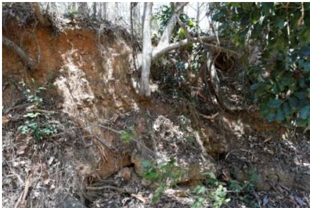
Plate 3 Bank erosion at KP418.35
