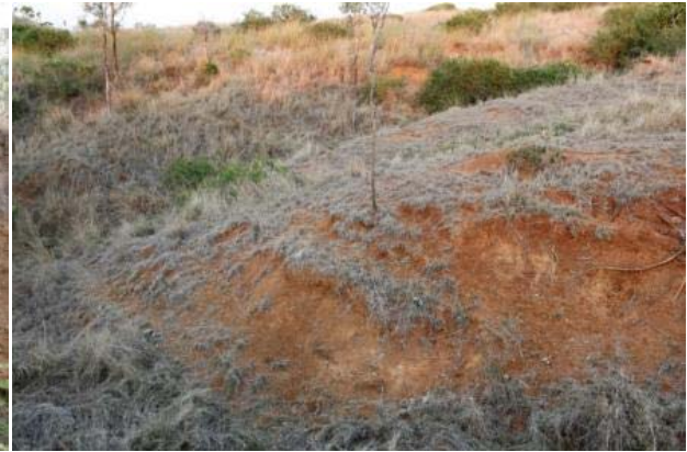
Plate 126 Minor erosion at drainage feature at KP402.47
