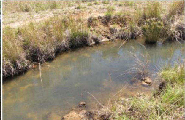
Plate 79 Ponding at KP 366.82
