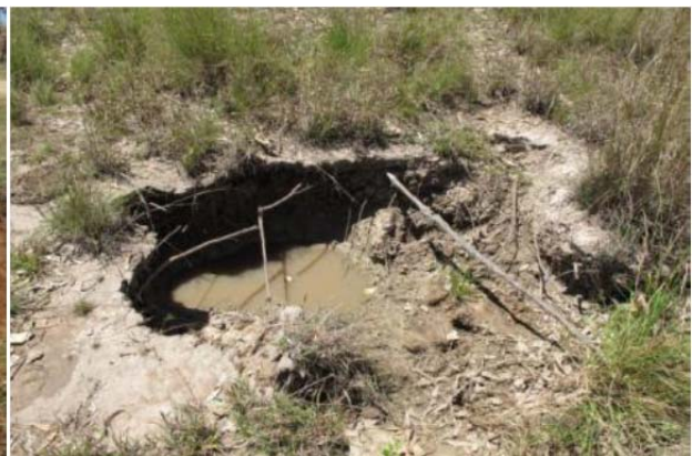
Plate 86 Sink hole in RoW at KP353.44
