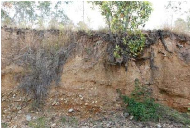
Plate 125 Creek bank erosion at KP398.06
