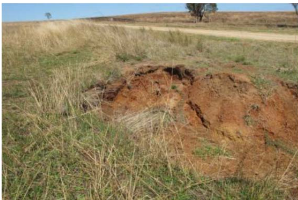
Plate 85 Erosion on side of pipeline at KP355.6
