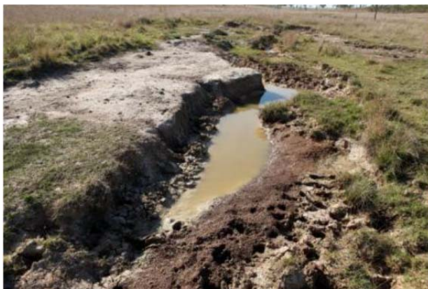
Plate 97 Erosion point at KP374.2
